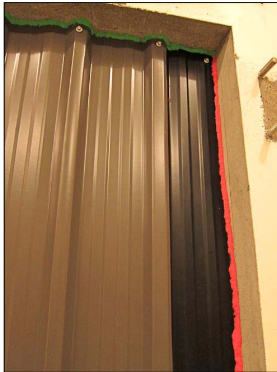
Figure 1: Sealing compound around the edges of the cladding to prevent sound leakage around the edges of the cladding.
