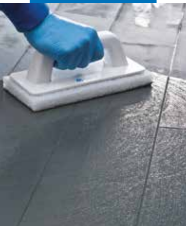
Cleaning the joints with a Scotch-Brite® pad (when the product is semi hardened)
