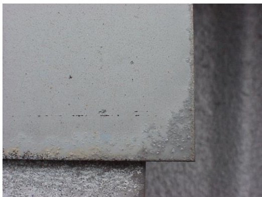
Under film corrosion on a coil coated section of galvanised steel. Exposed on GI roof for 15 years.
