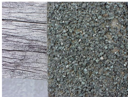
Edge of Al Zn steel acrylic tile. Exposed on GI roof for 22 years.
