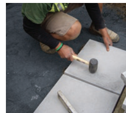
STEP 8. Gently tap paver down to desired level with rubber mallet. Joints should be approx 10mm wide at top of paver.
