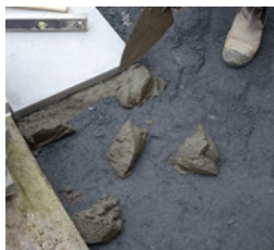
STEP 6. Trowel 5 spots of mortar mix onto base course. Then lay a strip of mortar where the next joint will be.
