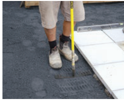
STEP 2. Compact base course to 60mm thick using feet or preferably plate compactor.
