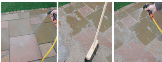
STEP 11. Wet the surface of the pavers and pour on the Premier P30. Wet the grout thoroughly and sweep into the joints. Only grout 4-5m2 at a time. Ensure the grout is a wet slurry!
