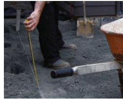
STEP 3. Check levels with tape measure. Your base course should be approx 60mm below the finished level of your paving.
