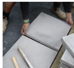
STEP 7. Gently lay the paver onto the spots (the mortar should squash down and spread out to 20mm thick. Use a sponge to wet the back of each paver before you lay.
