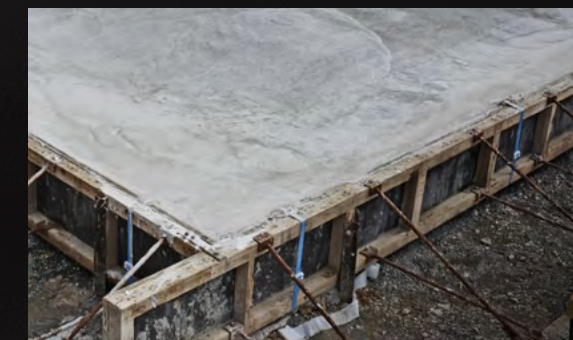
2 RibRaft® RaftMix® concrete is poured covering the angled top edge of the HotEdge® anchoring it into the slab.
