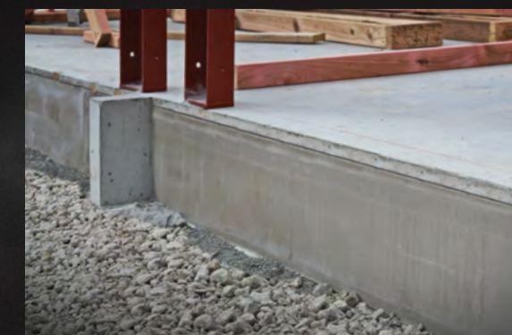
3 Boxing is removed, revealing a truly integrated, aesthetically finished thermal barrier. Once wall framing and cladding is fixed in place, for optimum service life and insulation, two coats of acrylic paint should be maintained to all exposed surfaces.
