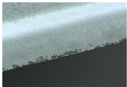
Underside of overlapped section edge corrosion
