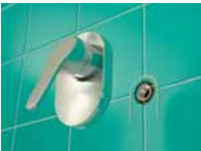
Run a bead of silicone sealant around the mixer unit on the tiles extending below the bottom of the pipe aperture.
